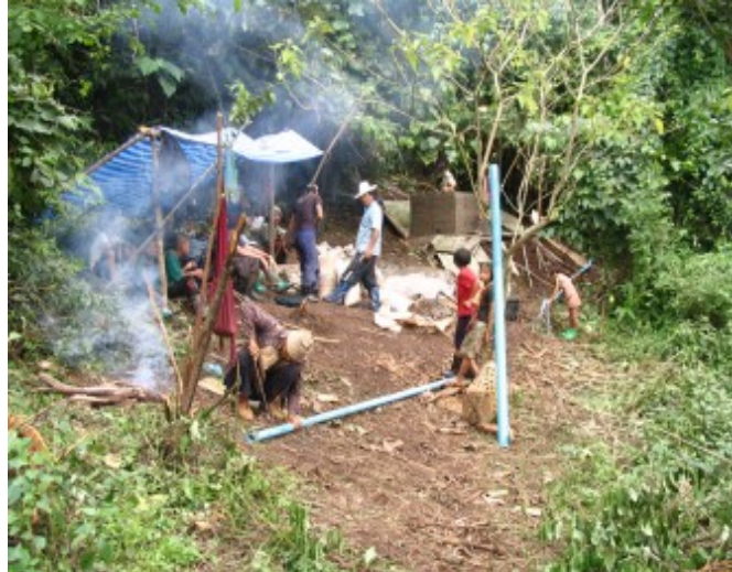
Water treatment installation, Northwest Thailand
